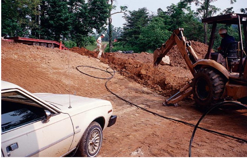
A buried service entrance requires a deep ditch—expect things to be quite messy.
