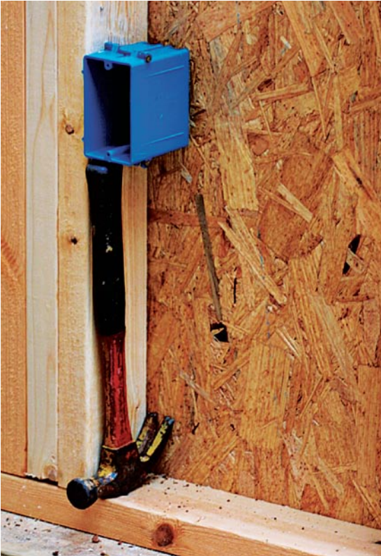
Using a hammer as a height gauge keeps all receptacle boxes at the same level and allows for quick installation.
