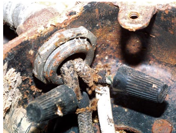
Even close up you can just barely differentiate the black (hot) from the white (neutral) conductor. The insulation on both wires is severely deteriorated and may break away if the wires are moved.
