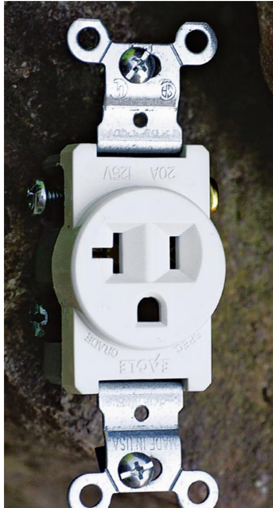
A single receptacle has only one place to plug in a load. Note the horizontal slot, which indicates that it is a 20-amp receptacle and capable of taking cords from heavy-duty, 20-amp appliances.
