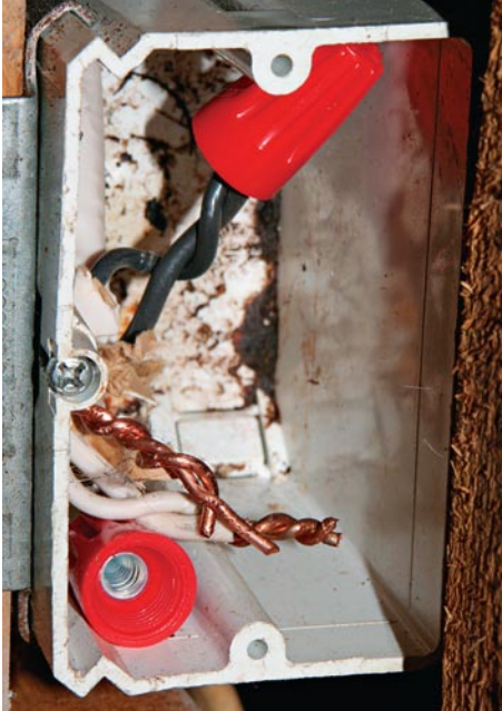
A wire connector has fallen off the neutral splice and the ground wire is pressing against bare neutral.
