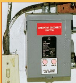
313 | History of Incorrect Connections
