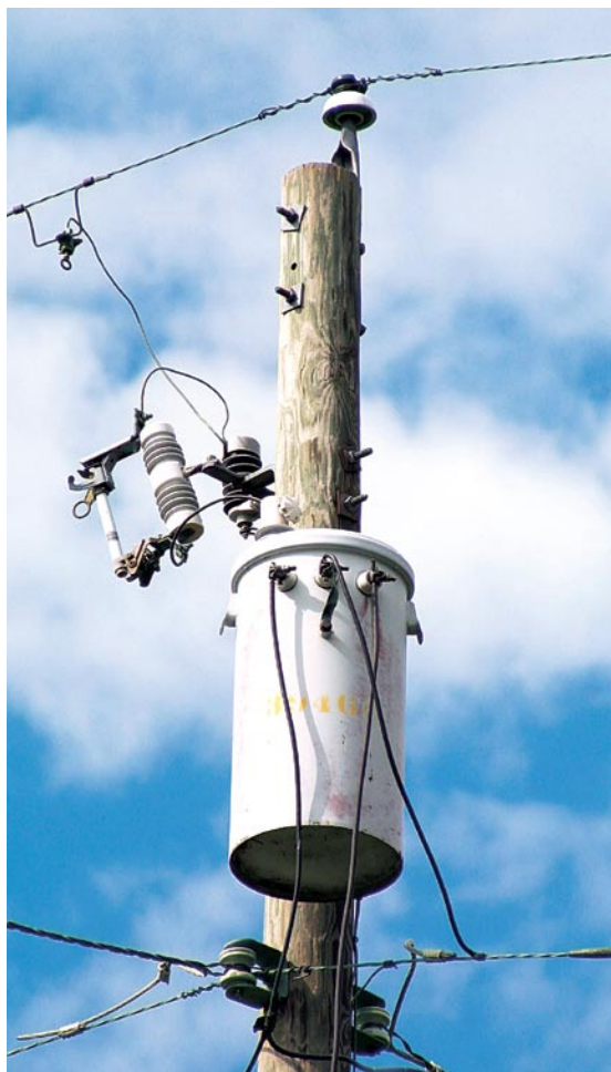
All electrical current originates from and comes back to the three side terminals of the utility transformer.
