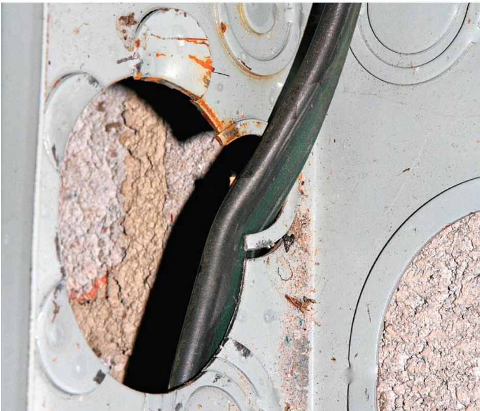
A panel entry without an NM clamp can cut or puncture a cable.
